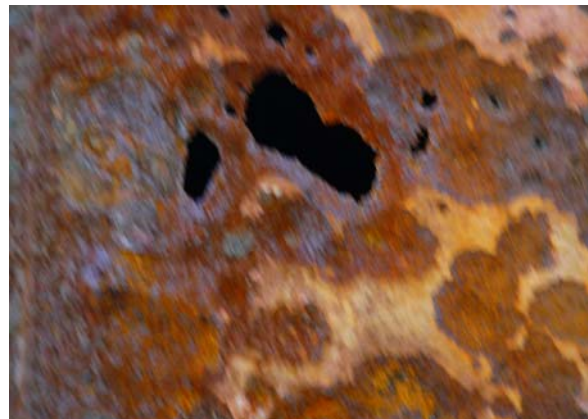
One of the many waterline rust holes.
