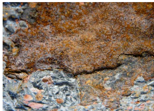
Flaky rust which is removed by chipping and needle gunning
